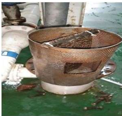
Gambar 5. Filter Seachast Rusak Sumber: kamar mesin MV. Dian Cordelia
